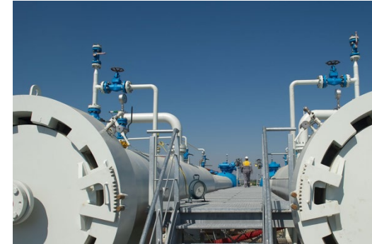
Automation/ Flow measurement
